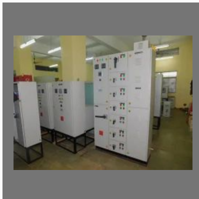
Motor Control Panel
