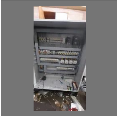
DB Control Panels
