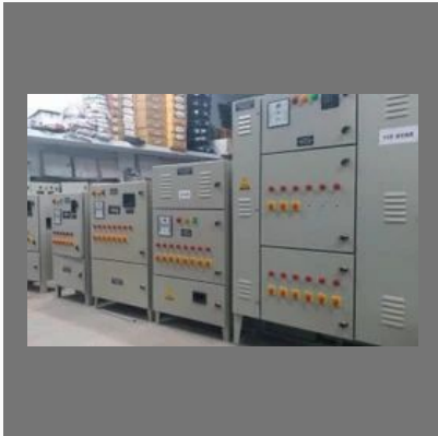
Apfc Control Panel
