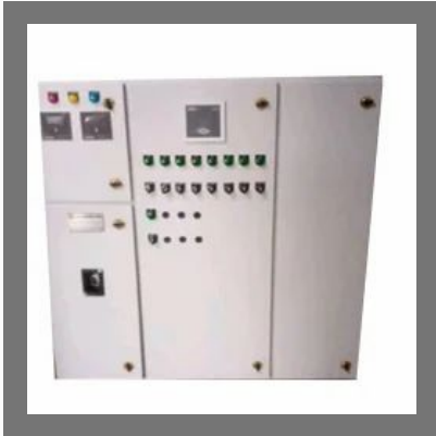
10HP PLC Control Panel
